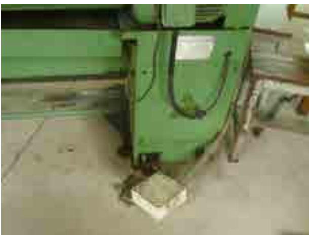
Electrical safety is not unsecured
