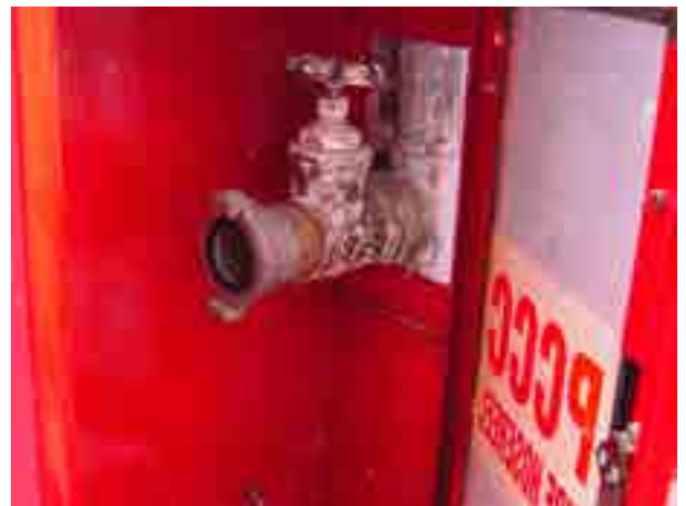
No fire fighting hoses, broken valves
