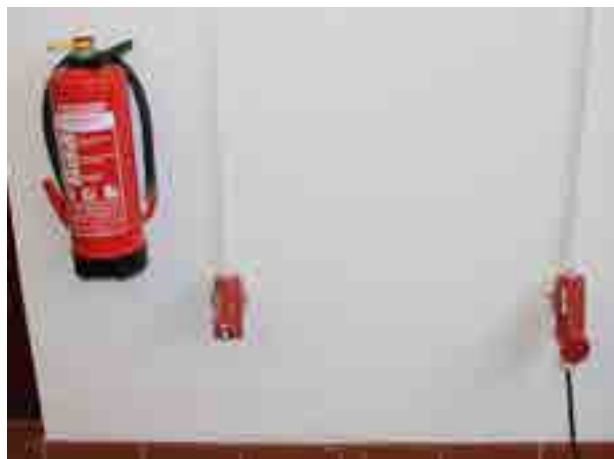
Electrical safety and fire protection
