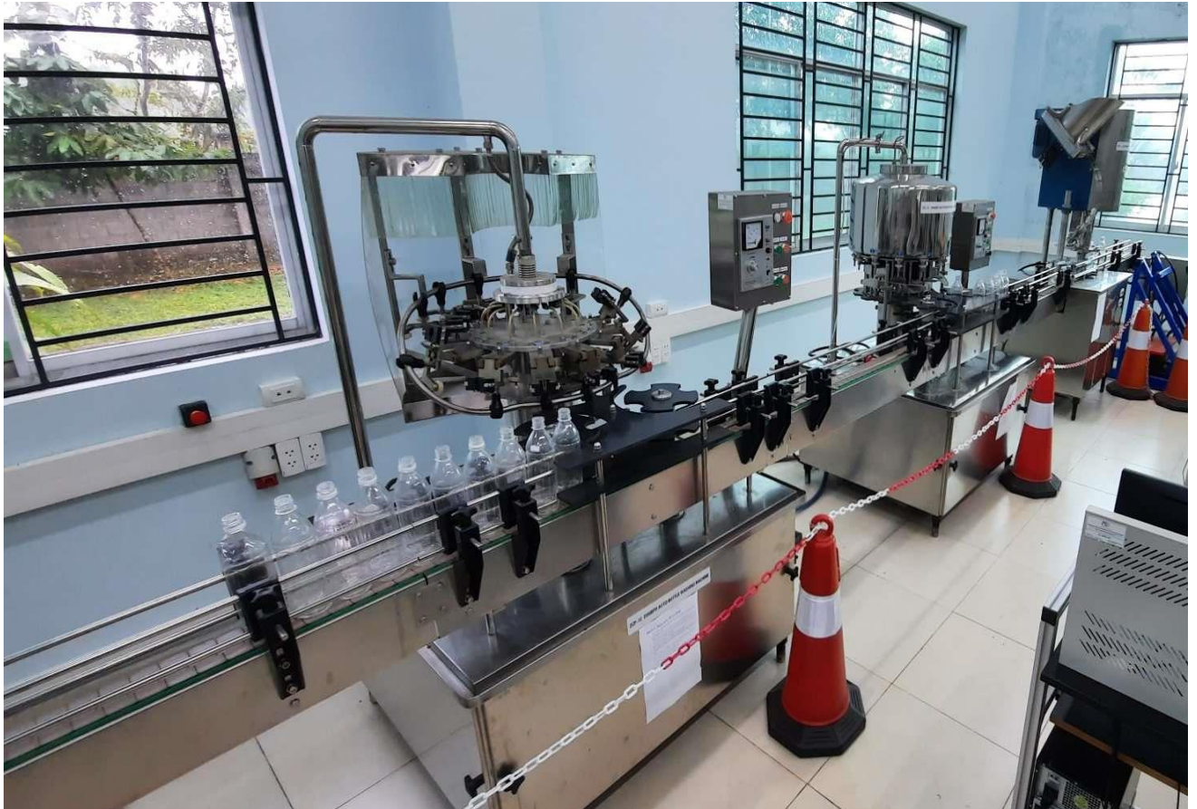
Figure 160: Bottling station full setup, cleaning(left), filling (middle) and capping (right)
