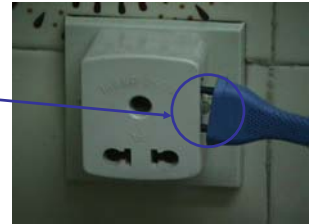
Power Plug loosely fitted
